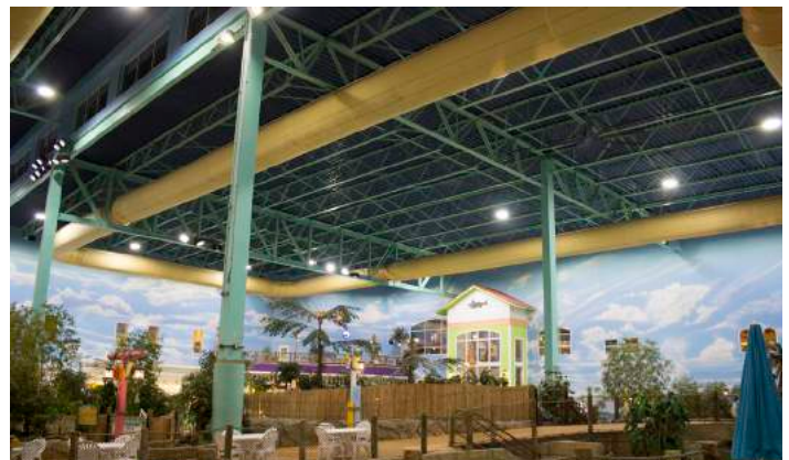
AFTER — 230W Phoenix LED Highbays
