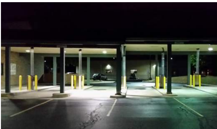
BEFORE — 250W Metal Halides
